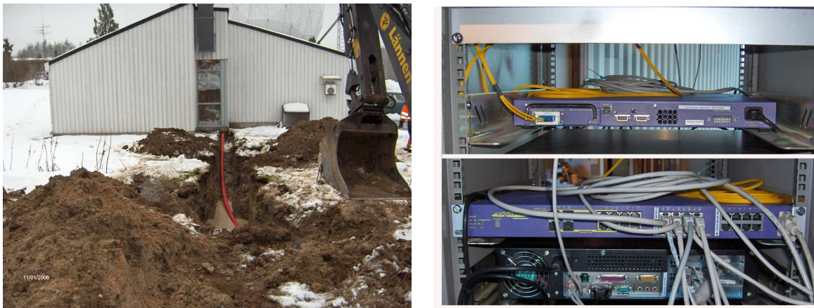
Figure 2: Last-mile fibre works (left) and equipment (right) at the 14-meter radio telescope in Metsähovi (Finland).
