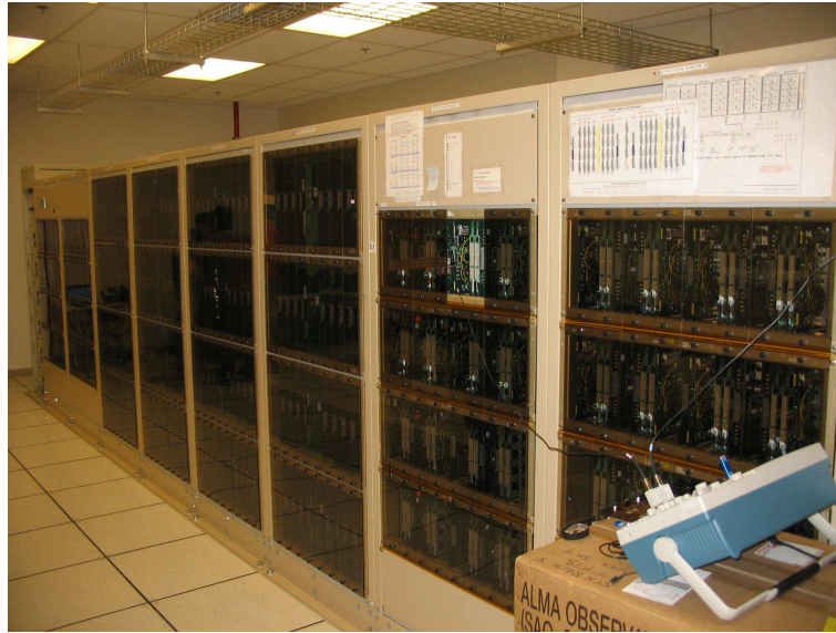
Figure 3: The 8 racks of the first quadrant of the 64-antenna correlator installed in a dedicated room at the AOS central building (5000 m). The 4 central racks contain the correlator cards while the 4 outer racks on each side of the central racks contain the digital filter cards and other station electronics cards. Heat dissipation from thousands of cards in the system is a difficult task at 5000 m because the air density is nearly twice less than at sea level.
