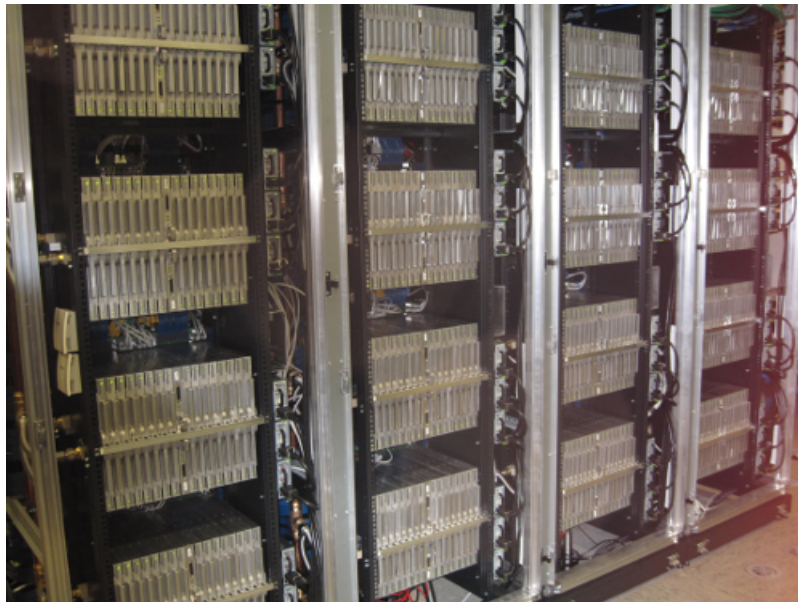
Figure 9: 4 QPACE racks installed at the Jülich Supercomputing Centre.
