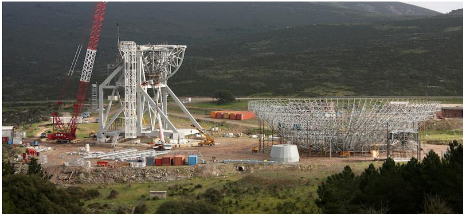
Figure 2 – SRT antenna still in two parts: the main dish, now on ground, will be raised soon on top of the alidade structure in a single lift procedure, which is a first in the world, for such a large and heavy backup structure.
