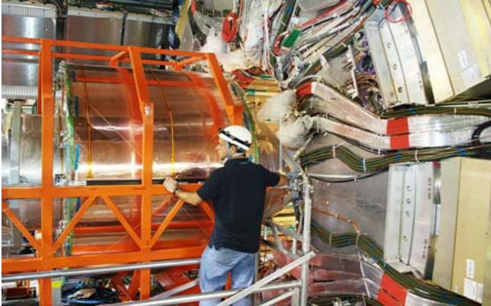
Figure 2 Barrel TRT and SCT installation into the ATLAS detector. Cable services take nearly all available space between the inner tracker and calorimeter.
