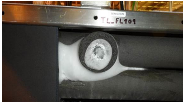
Fig. 3: Forming of ice at a spot in the cooling plant that is improperly insulated.
