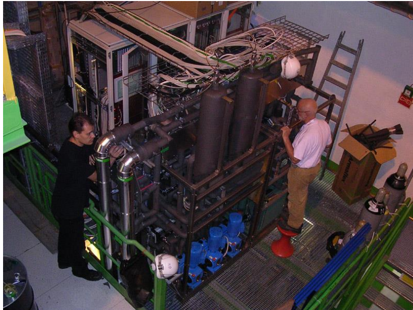
Fig. 4: Picture taken during the installation of the cooling plant in the radiation free zone. On the front left the CO 2 plant with the 3 CO 2 pumps (blue) and the 2 accumulators (grey) on top. The freon plant with the water-cooled and air-cooled chillers is on the front right. In the back the rack with the PLC, PLC-screen and other control electronics.
