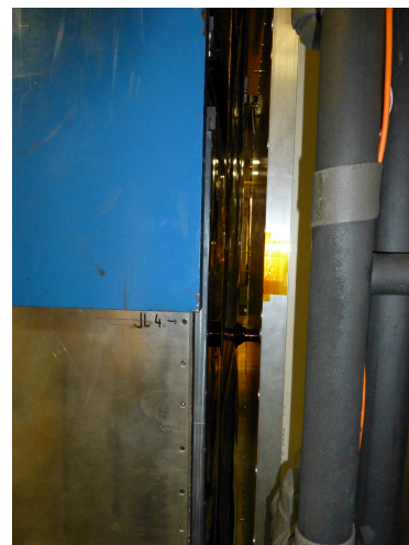
Figure 3: The VHCC between RICH1 and TT installed for the 2015 run.
