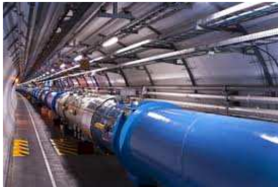
Figure 4: A view of the LHC tunnel and the superconducting magnets.
