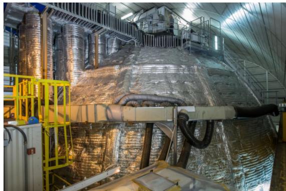
Figure 4: External Borexino appearance after TIS installation in early 2016.
