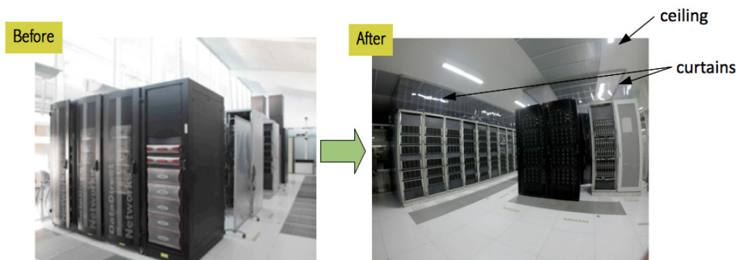
Figure 5: PIC main computing room before (left) and after (right) completion of hot/cold air separation and confinement.
