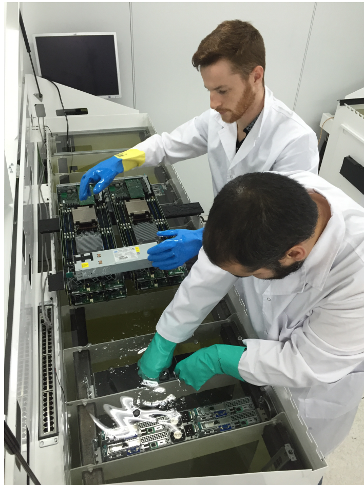
Figure 6: PIC members installing the first CPU units into the oil tanks from Green Cooling Revolution, at the beginning of 2016.
