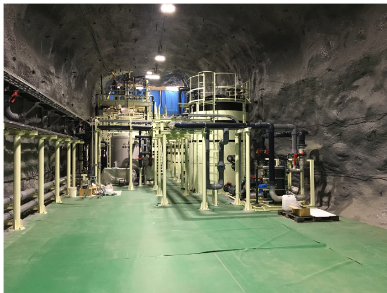
Figure 4: A new cavern was excavated in April 2016 for the new SuperK-Gd water system new the SK site. Installation of the new water system started (piping, Gd dissolution, controlling system, etc). In the next months other relevant parts like the band-pass system will be installed.
