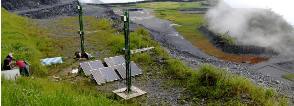
Figure 4. TAROGE-II tower structure. TAROGE-II includes three towers structure and each tower carry two dual-polarized LPDA antennas with a 2.5 meters spacing. This figure shows two towers and a 800W PV array system are placed in between of them.
