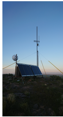
Figure 9: One of the constructed tower (SCCT). This tower is located on the top of a hill about 60 m high above surrounding ground level.
