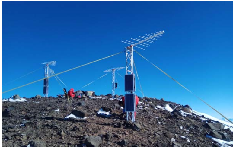
Figure 4: The prototype station installed on the top of Mt. Melbourne (March 2019)
