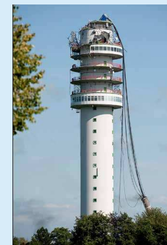
Figure 3: The unfortunate and collapsed transmission tower in Hoogersmilde on the afternoon of July, 15th 2011. Obviously, no radio interference was noticeable afterwards! © Jürgen Morawietz
