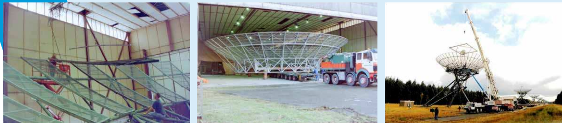
Left to right: 1994 removal of outer-panel of RT5. 1994 reflector ready for transport to RT5. 1998 November, lifting of last revised reflector on RT0
