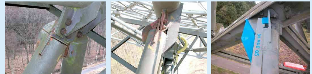
Left: RTC in 2004 connection to declination axle is completely broken. Middle: Connection to the declination axle, re-welded and reinforced on all 14 telescopes. Right: additional strengthening of the tube counterweight construction now on 12 telescopes
