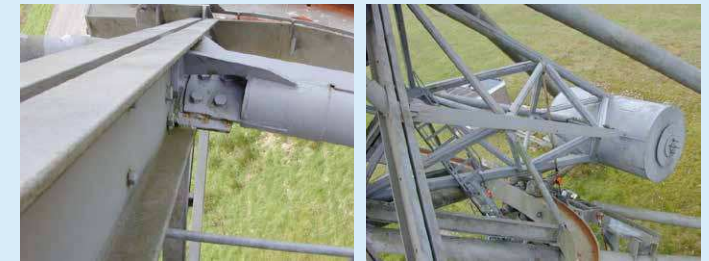
Left: A repaired tube with an additional strengthening member added. Right: Hour-angle counterweight construction, with all members doubled in steel on all 14 telescopes.
