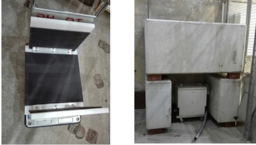
Figure 2: Protection of PLC CPU for the magnet system. Right side : The CPU is installed in the polyethylene box which is covered by the concrete blocks. The front concrete block, which is not shown in this picture, is movable to access the CPU easy. Left side : The top cover of the polyethylene box with the boron-carbide sheet.
