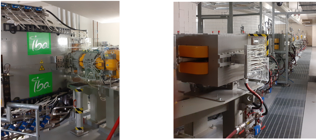
Fig. 2.2: The the cyclotron output point (left) and the beam distribution line (right).
