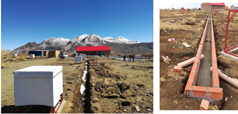
Figure 4: Photos of the ALPACA site. (Left) SDs, central hut and cable drain in preparation. The mountain behind the hut is Chacaltaya. (Right) A cable drain reinforced with bricks and concrete.
