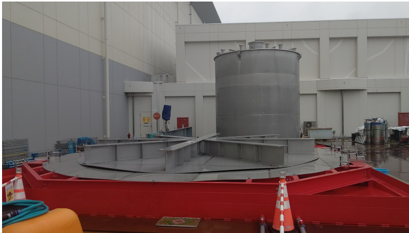
Figure 3: The status of s.s. tank construction of the JSNS 2 -II as of 17 December 2021. The inner s.s. tank can be seen in the back, while the base of the detector and the support structure of the outer s.s. tank can be seen in the front.
