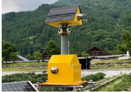
Figure 5: Outdoor Camera House Shelter.
